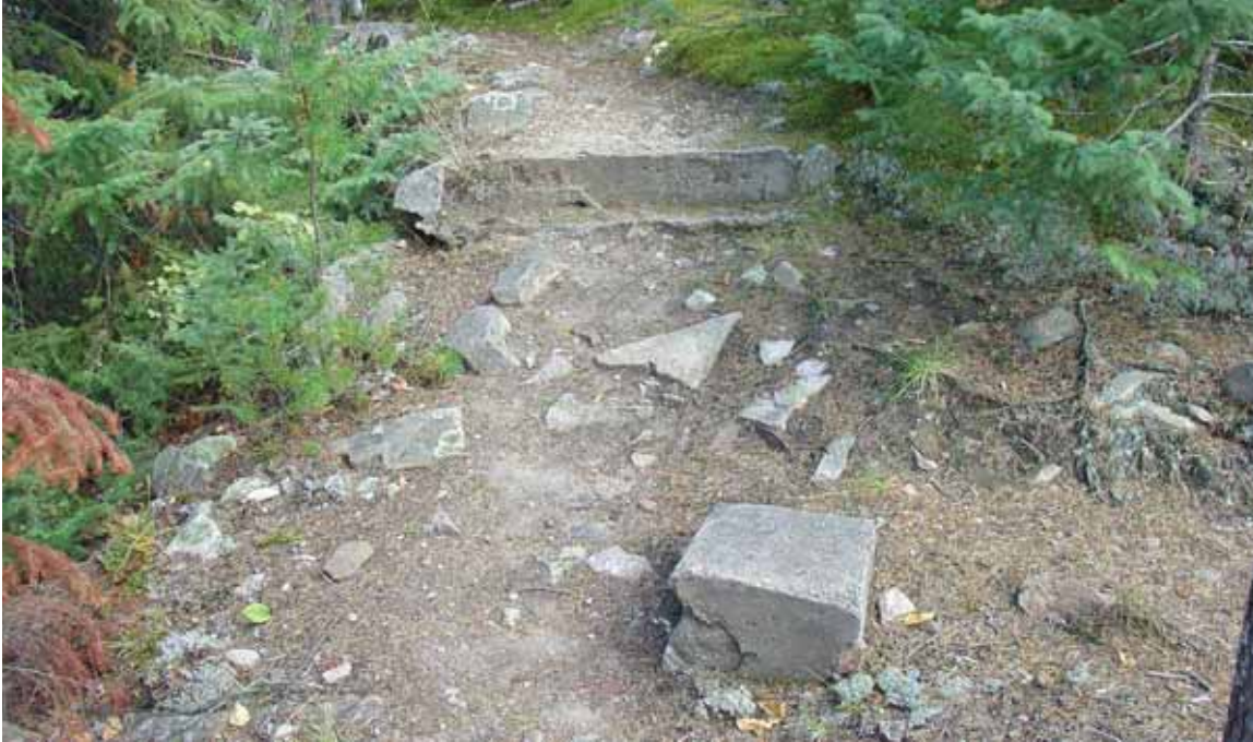
Figure 4- 35: Threshold (background) and square concrete cabin foundation post at Carey Cabin (#1 Cabin), August 2012 (source: QEA)
